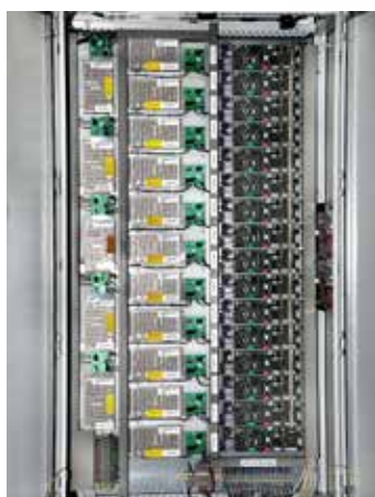
Control cabinet with power packs and zone masters that coordinate transports within the respective zone.
